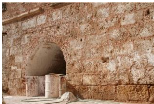
Fig. 13- Materials and constructive typology " opus quadratum and opus testaceum " of the mosque ©Abdessemed-Foufa 2010
