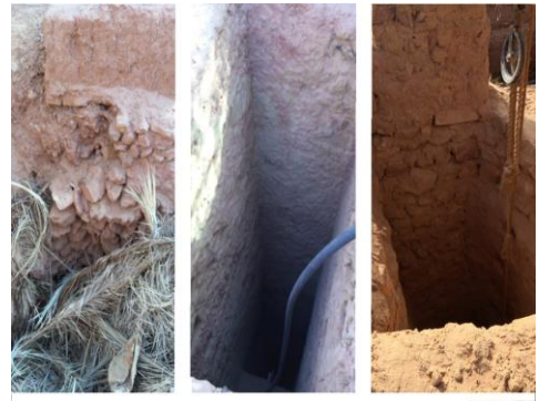
Fig. 5- Constructive techniques of Tala Aougrount stone wells: monolith and masonry limestone and sandstone. (Illili Mahrour, 2016).
