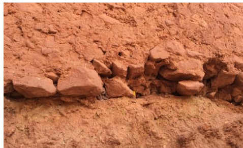
Fig. 14 - Constructive stone detail from the western wall of Tala Aougrouit old fortress "El Guesba El Guedima" (Illili Mahrour, 2016)
