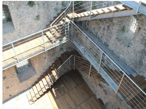
Fig. 3 Belcastro (CZ), the interior part of the Donjon. Ramps and walkways during the construction.
